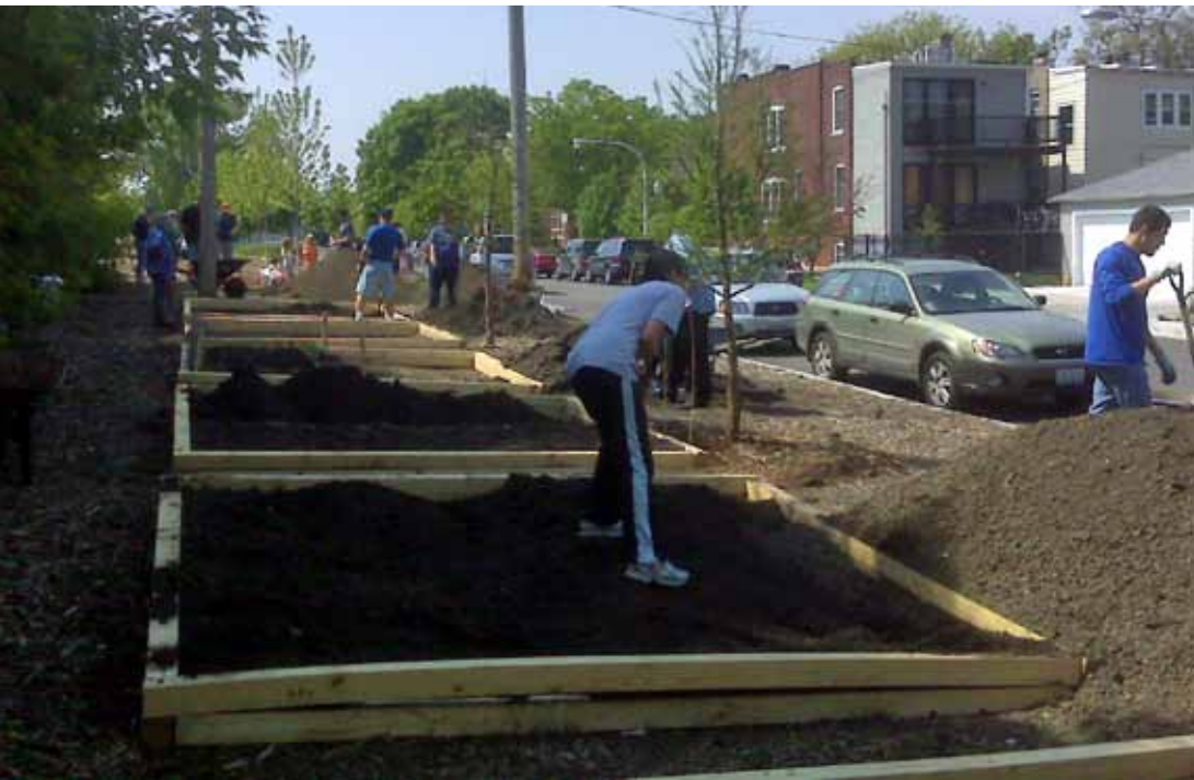
The space along railroad tracks can be turned into prime garden real estate, but be sure to get a green light from your alderman, the railroad (in this case Metra), and then make sure the soil is safe. When the members of the Ravenswood Fellowship United Methodist Church learned that the space they wanted to use for vegetable growing was contaminated with “anthracitic compounds,” they went to Plan B and built raised beds instead.
